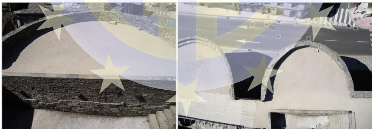
Figure 10: images of the parapet of the walls at the Miñá gate from the UAV camera.
